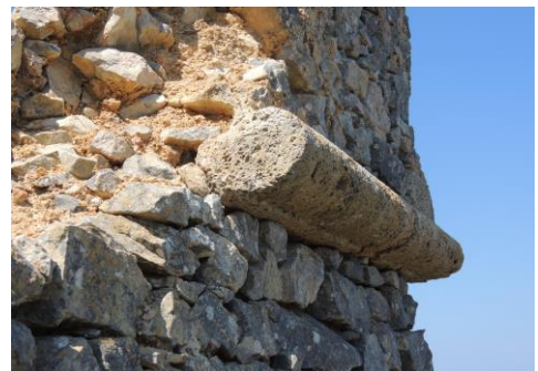
Fig. 6 – Tower of Capodomo: the cornice made of Cavernous Limestone and the dressed stones made of calcitic grey marble
