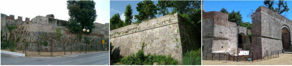
Fig. 1- Images of the only three existing bastions of the city walls of Pisa. On the left, the Parlascio Bastion; in the centre, the Barbagianni Bastion; on the right, the Stampace Bastion
