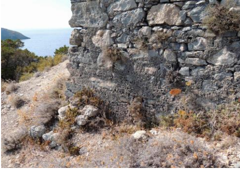
Fig. 11 – Tower of Calamoresca: residues of plaster near the base.
