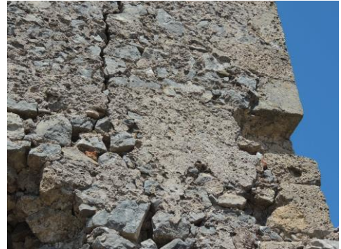
Fig. 5 – Tower of Capodomo: plaster residues
